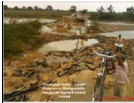
Bridge damage Dharwad district – 5 th October 2009
